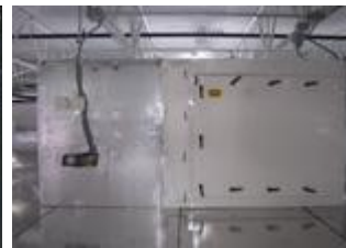
Blower For Clean room
